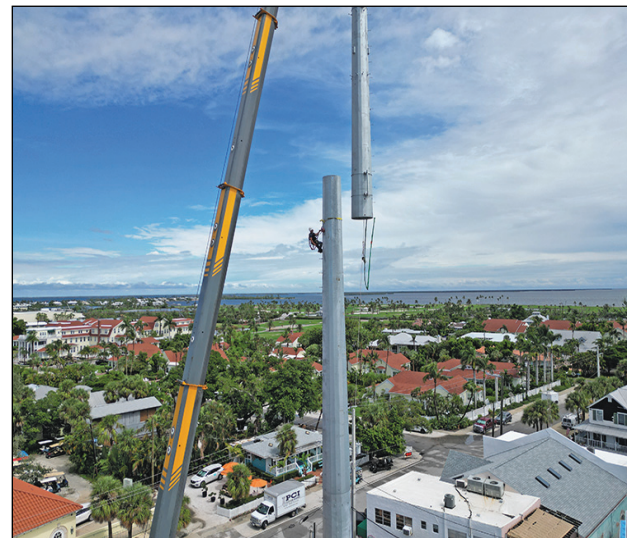
■ Like a camel through the eye of a needle, T Steele Construction got it sorted and done.
